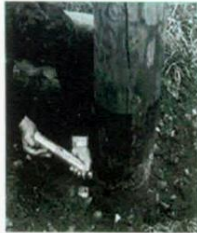
Measurement between pole and ground
